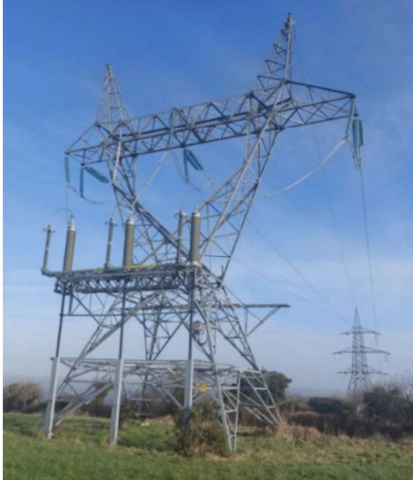
Figure 2-9: Line Cable Interface Mast (LCIM)
